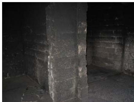
Figure 3 Measurement room interior
